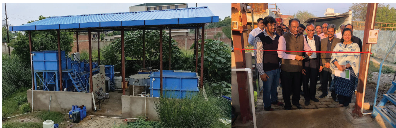
Figure 4: 20 KLD Plant (Left) inaugurated by Director General (DG), NMCG on 17th February 2023
